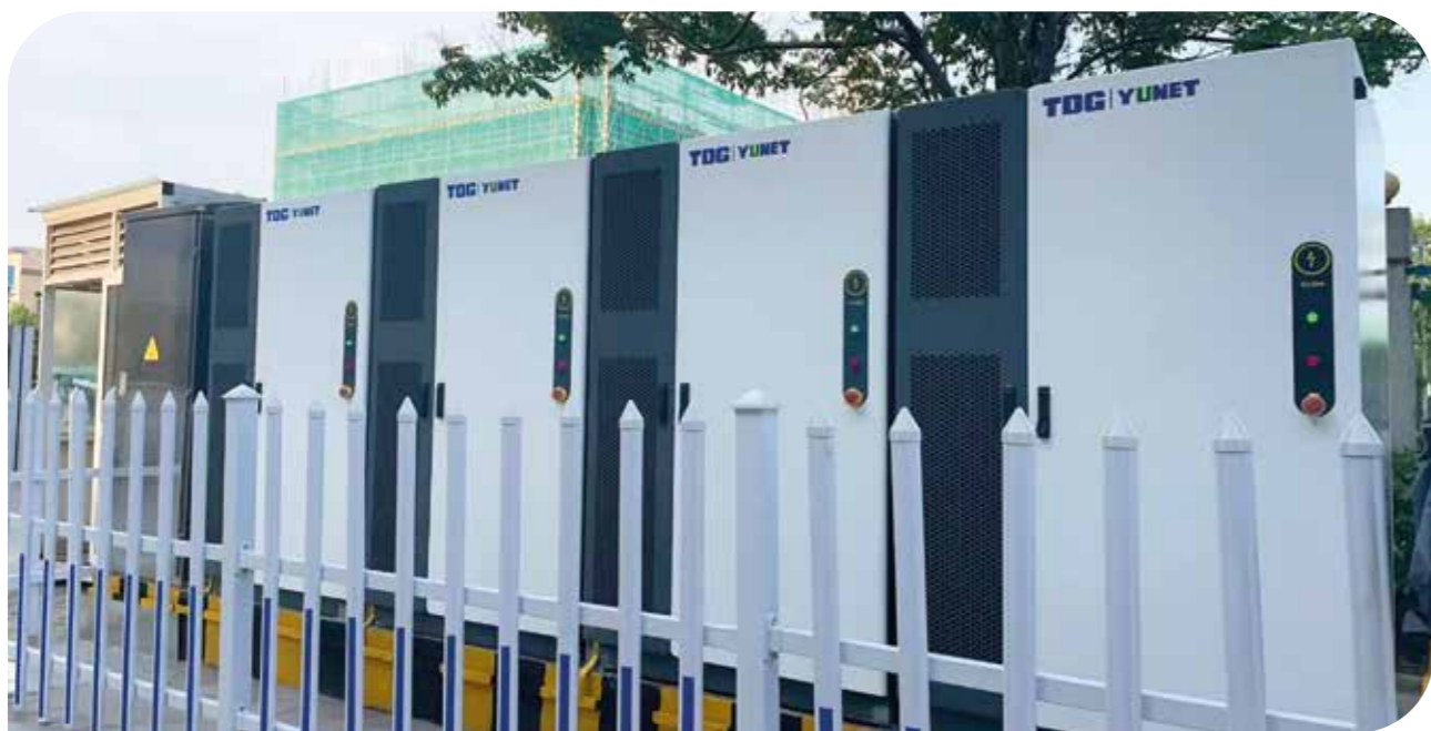
6 Modelo: HELIOS UE-L232 Potencia instalada: 925 kWh Haining, Zhejiang, China
